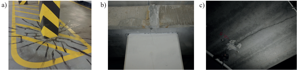
Fig. 6. Scratches in the ceilings (a), binders and columns (b) and cracks in the floor slabs (c)
