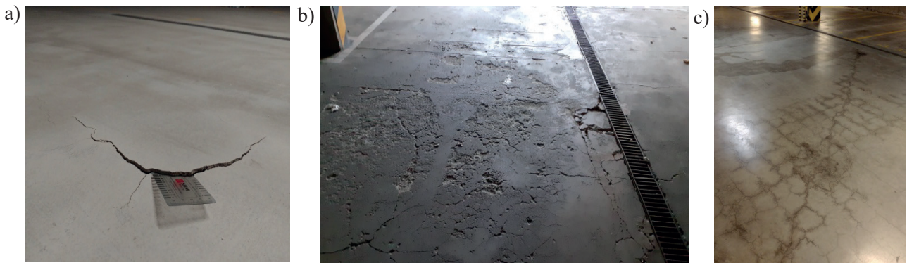
Fig. 4. Damage to the usable floor layer: detachment of the resin coating (a), extensive concrete chipping (b), surface scratches (c)
