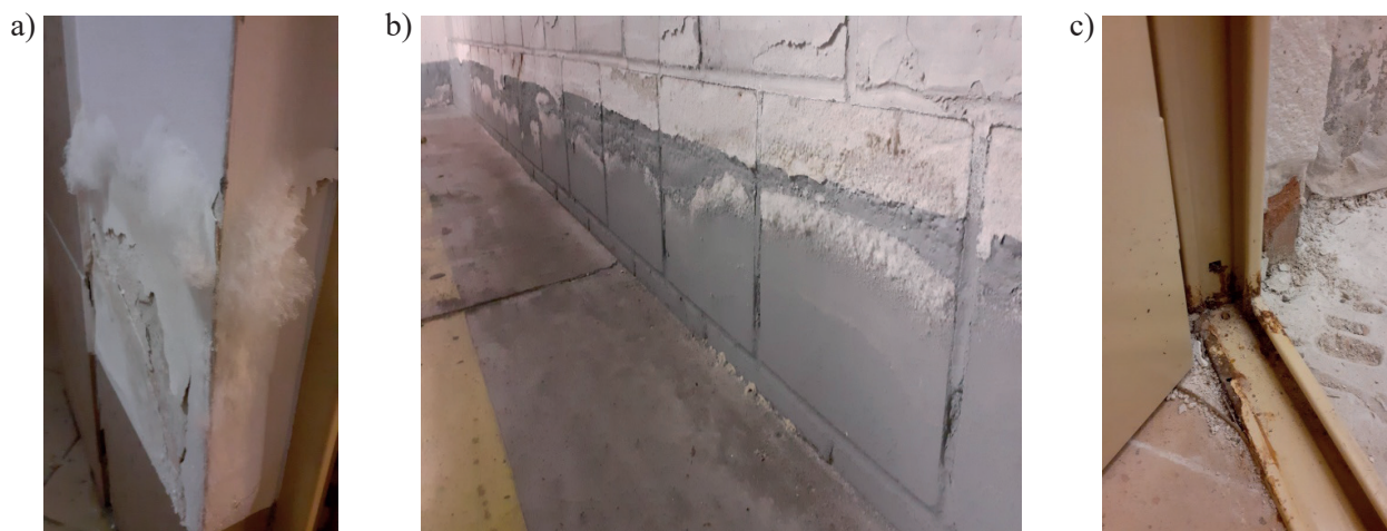
Fig. 1. Water rising at the joint between the floor and walls (a, b) and corrosion of steel elements (c) exposed to permanent moisture
