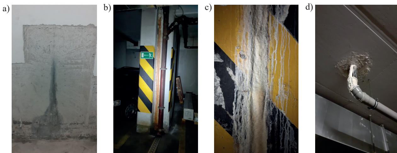
Fig. 2. Leaks through external walls (a), expansion joints (b, c) or installation penetration points (d)
