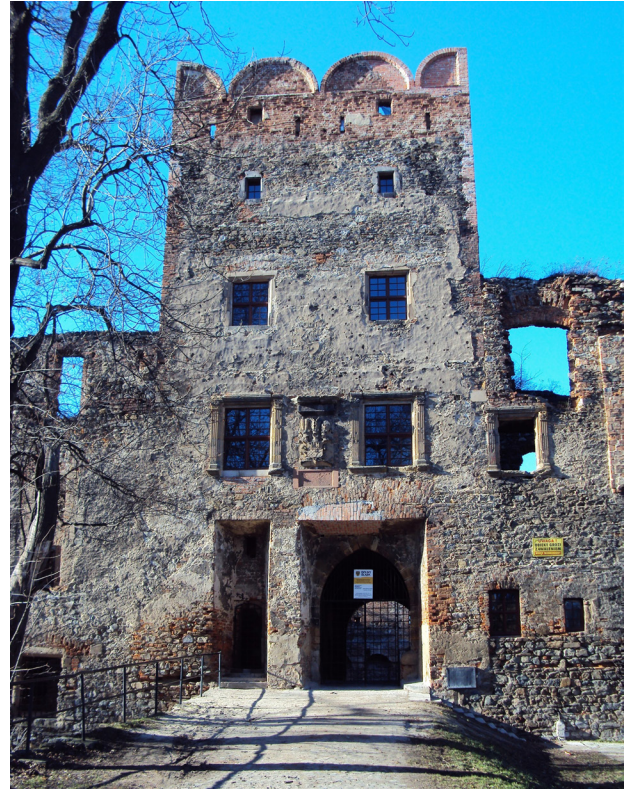
Fig. 10. The central part of the facade of the castle in Zabkowice Śląskie (photo by B. Czechowicz)
