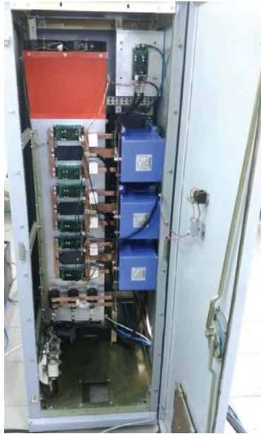
Fig. 7. View of the laboratory three-phase three-level 55 kVA inverter
