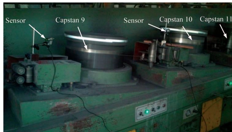
Fig. 2. Sensors positions for measuring the capstans speed
