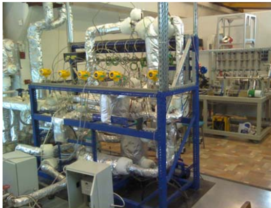
Fig. 16. The picture of pipeline from the evaporator
