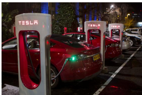
Fig.1 Tesla Supercharger Akkerhage, Ghent, Belgium.
