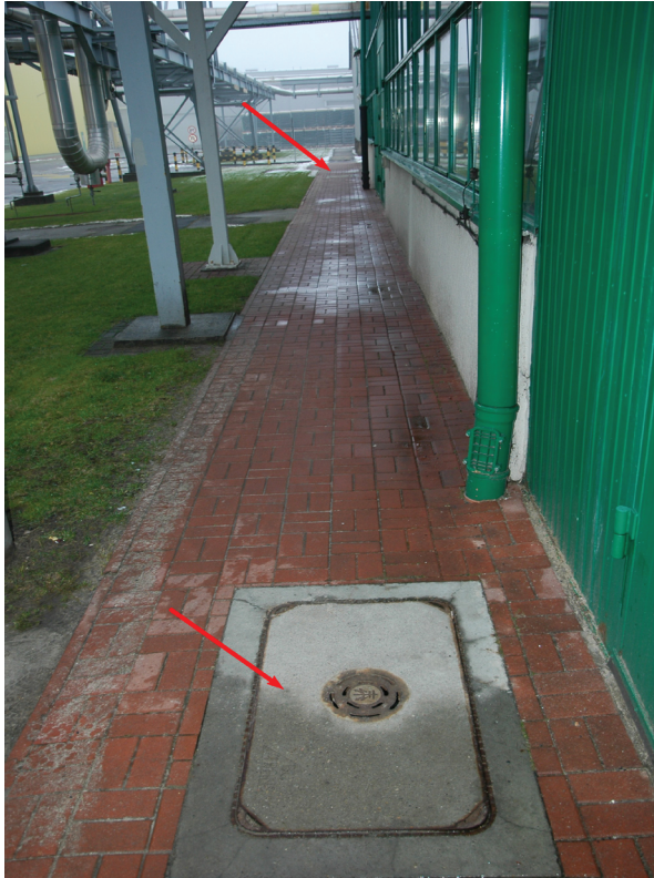
Fig. 3. Cable line between wells (structure), placed in the ground along the wall of the compressor building
