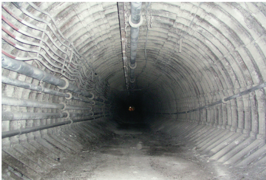
Fig. 4. Excavation corridor with roof support (mine working), where the suspended railway is located (technical equipment), drainage and fire protection pipeline, as well as power cables (technological installations)
