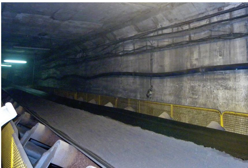
Fig. 2. Transportation tunnel with lighting installation (structure), where a conveyor belt (technical equipment) is located and cable lines (technological installations)
