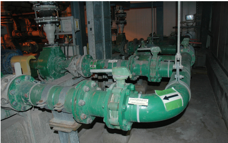
Fig. 1. Pump house with lighting installation and foundations under machinery (building), where pumps are located (technical equipment) and pipelines (technological installations)
