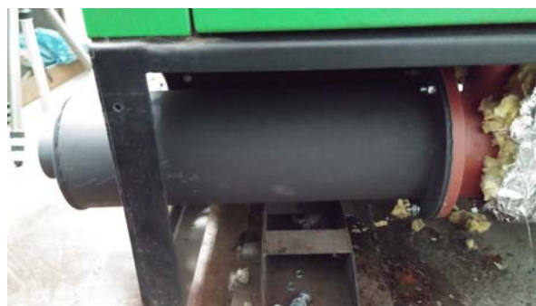
Fig. 13 The muffler mounted on the heat exchanger
