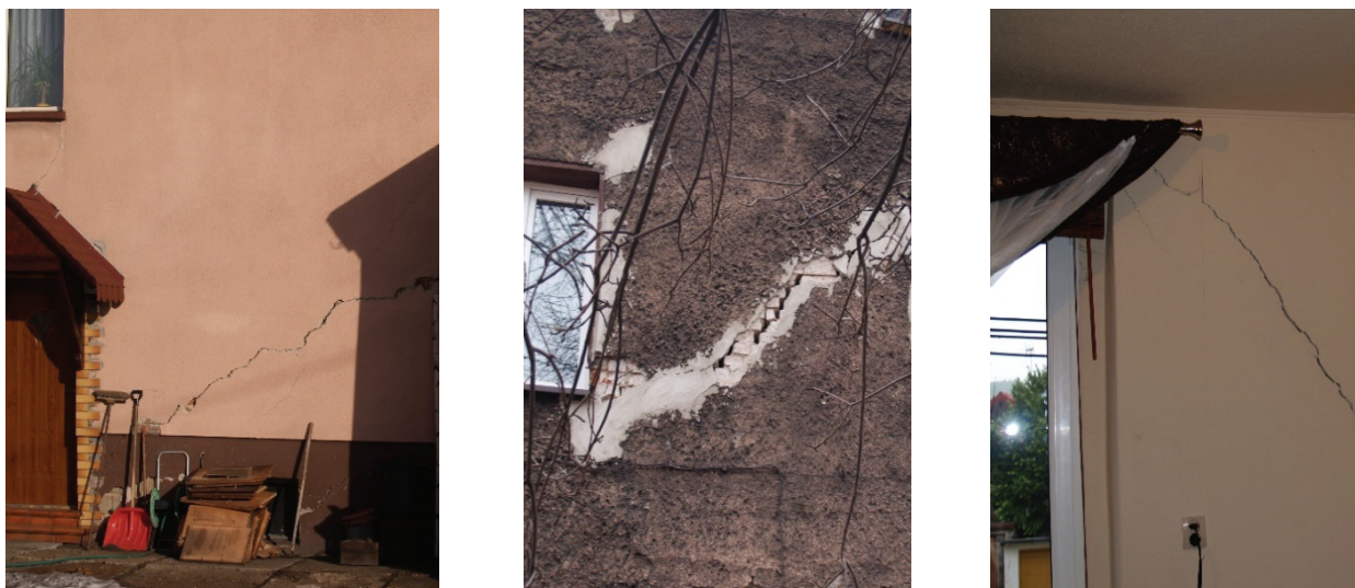
Fig. 1. Examples of damage to buildings subject to additional loads resulting from land surface uplift, analogous to those described in [26]
