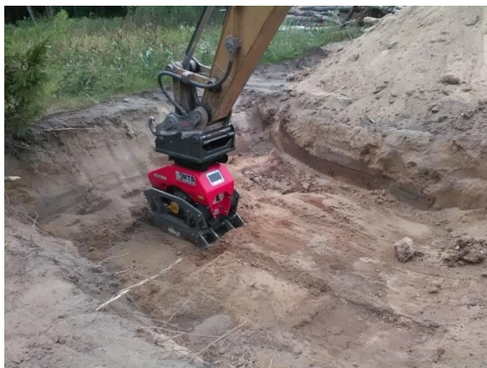
Figure 6. Compaction of the soil layer in the excavation by means of a hydraulic plate compactor
