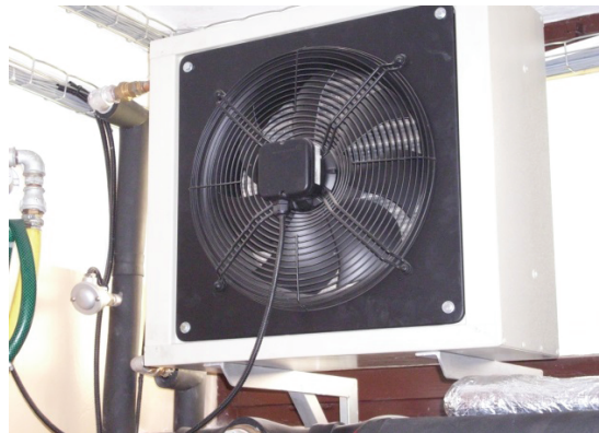
Fig. 1. Air-to-glycol heater in the installation owned by the Geoenergetics Laboratory, FDOG AGH UST (photo by A. Złotkowski)
