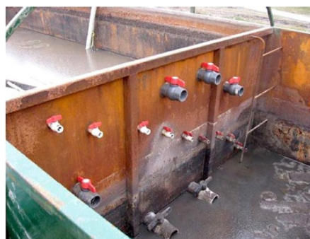
Fig. 3. Settling tank with visible corrosion caused by microbial contamination [12]
