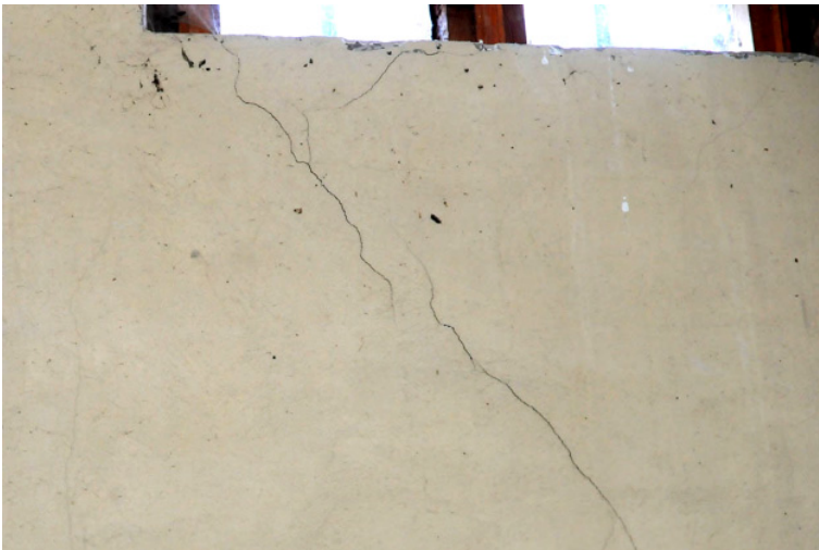
Fig. 11. A scratch, 1 mm wide (the largest in the building) extending from the door lintel to the window above the western entrance (unchanged). Source: Own study
