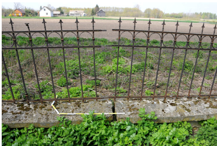
Fig. 12. One of the cracks in the construction of the fence around the church building on the north-east side (present situation).
