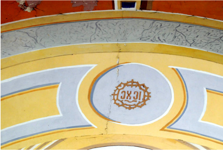
Fig. 10. Scratches of the arch crowning the nave from the side of the main entrance (unchanged). Source: Own study
