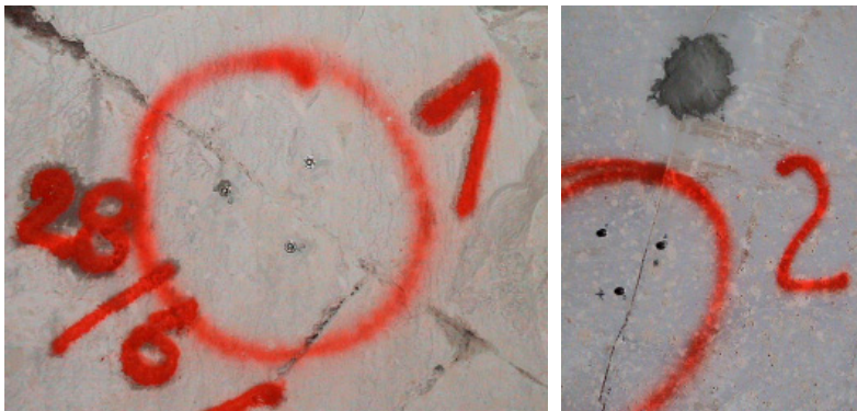
Fig. 10. Visual (cement seal) and manual (three screw system) measurement of the displacements of open dikes within safety pillars
