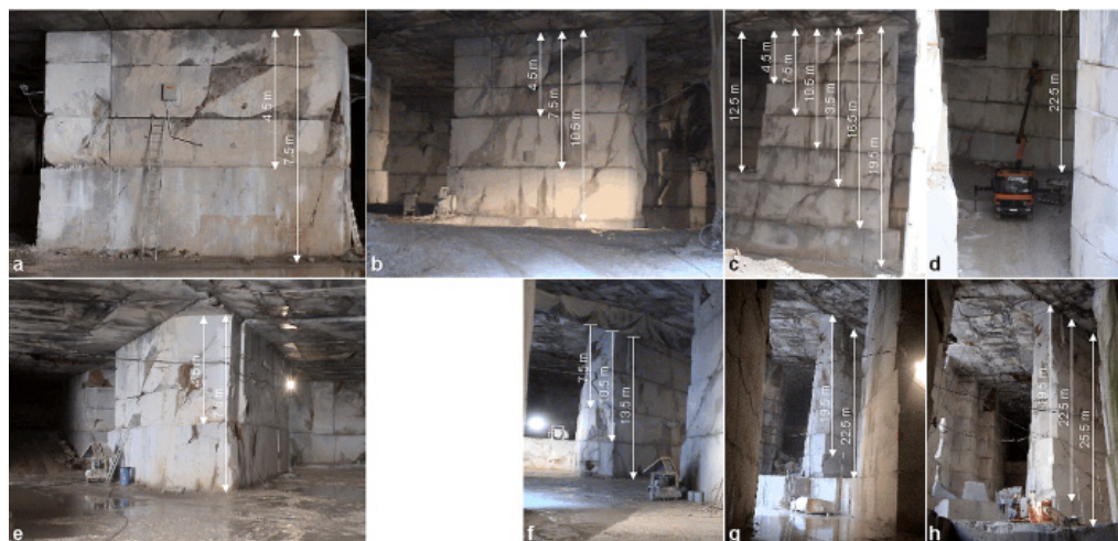
Fig. 8. Deepening (from 4.5 m (a) to 25,5 m (h)) of the high safety pillar SP02 (cross-section area 72 m 2 ) in Lipica II. quarry
