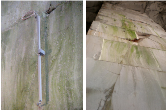
Fig. 9. Vertical EL beam gauge installation on the high safety pillar VS3 in Lipica II. quarry
