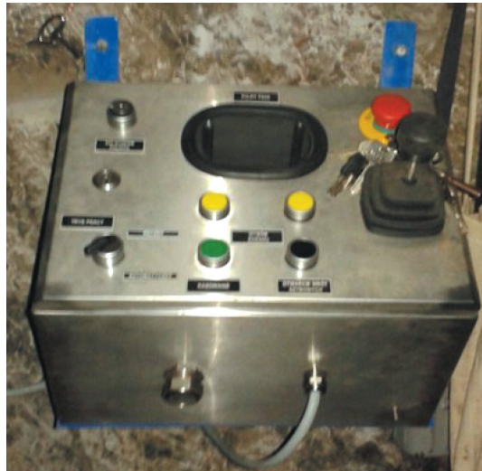
Fig. 4. Control panel view
