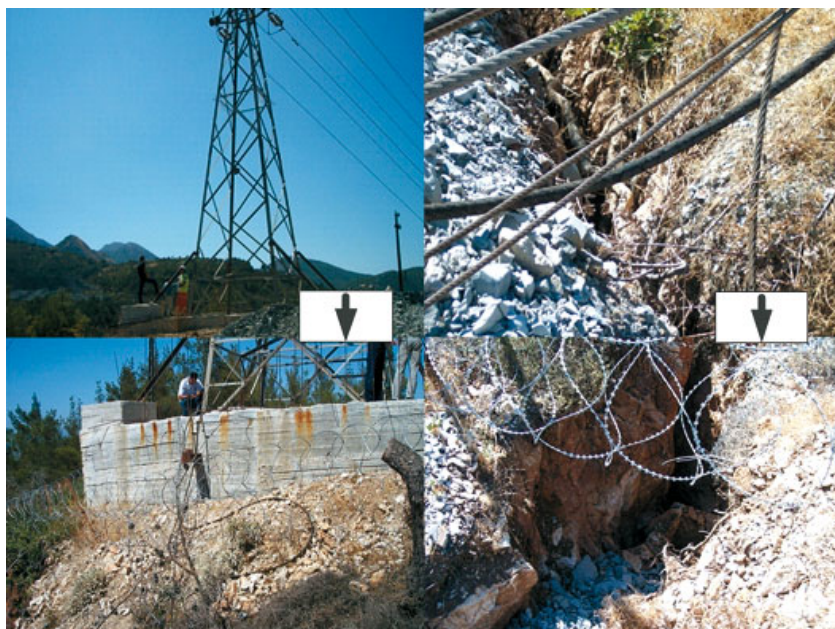
Fig. 7. Preview of subsidence effects on Pylons (No: 18-19)
