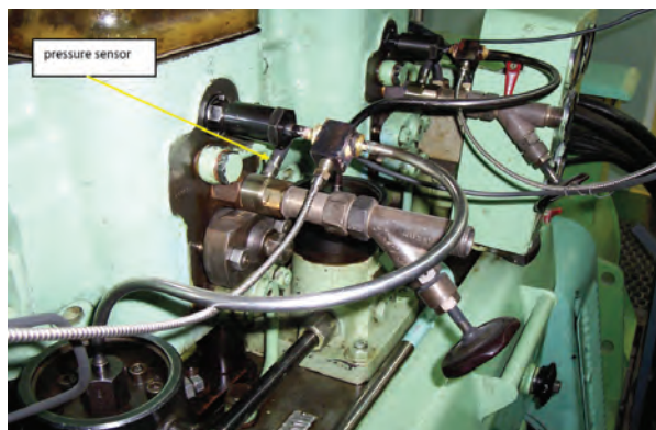
Fig. 1. Pressure sensor Kistler installed in indicator cock
