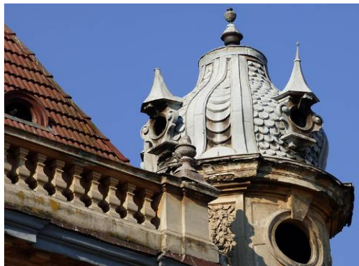
Fig. 21. Covering of the roof with so-called 'moulding iron roof tiles'. The tower of the building on Soborna Square. Photo by Sergii Lieonov
