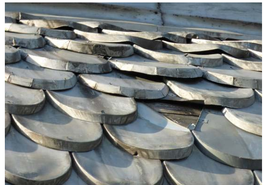
Fig. 22. The fragment of the Covering of the roof of Sacrament church with so-called 'moulding iron roof tiles'. Source: photo by Sergii Lieonov
