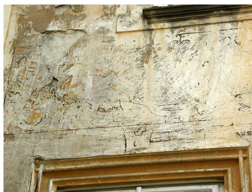
Fig. 5. Fragment of façade painting of Schulz brothers' mansion. Ochre background and black outline. Source: photo by Sergii Lieonov
