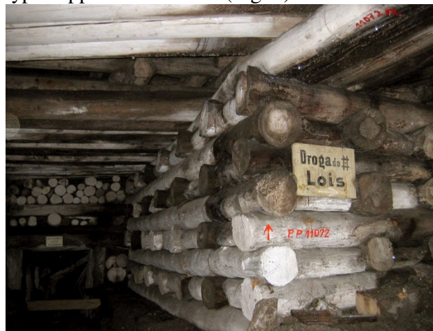
Figure 5: Original crib support (1857) at the crossing of the Gębaliński and Lois-2 galleries (photo T. Wieja)
