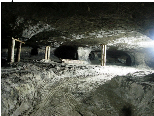
Figure 4: An example of a modern simple support structure - props with cross binding, underground tourist route Nagórzyckie Grottos (photo T. Wieja)
