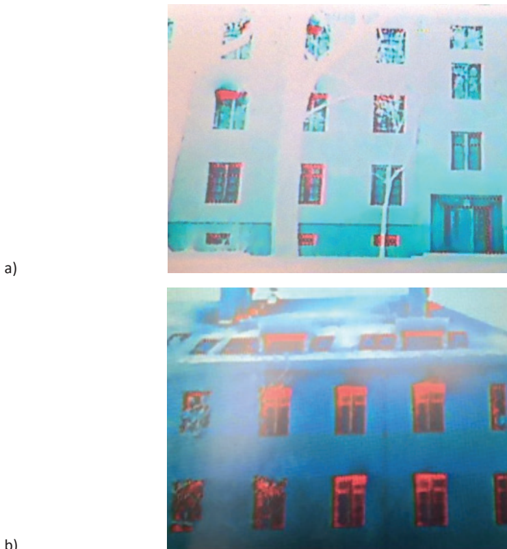
Fig. 1. View: a, b) building thermogram made with the use of UAV Source: Author's own study.
