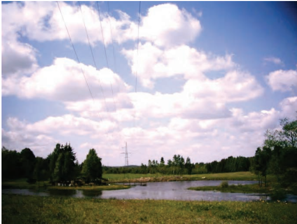
Photo 1. Power line located in a wetland with humus soils and high moisture content
