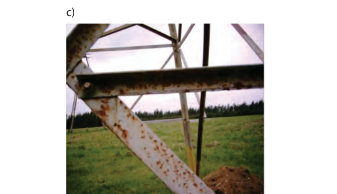
Photo 5. Discontinuities and areas where the coating is thinner: a) underpainting, b) overpainted inclusions and weld spatter, c) insufficient coating thickness in a given corrosive environment
