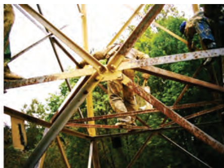
Photo 8. Improper seasoning of coatings applied at the construction site (application of a plastic film over a non-dry coating) leading to coating damage and long-term penetration of solvent from the topcoat into the primer coat
