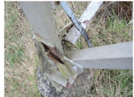
Photo 15. Corrosion in unprotected cracks
