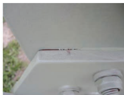
Photo 7. Lack of joint protection leading to joint corrosion and detachment of coatings around the joint
