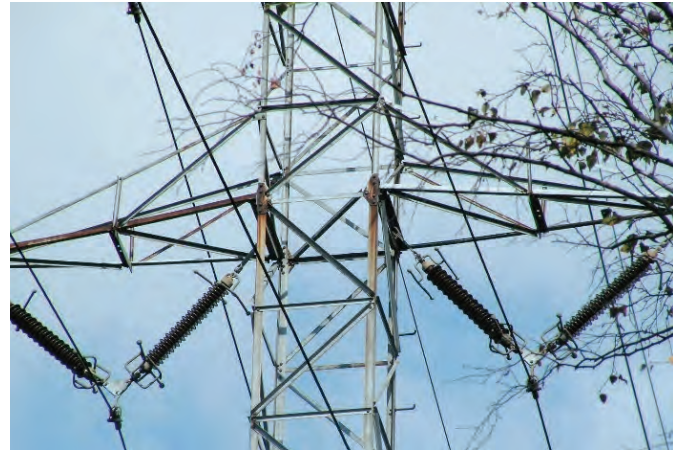
Photo 2. Corrosion of galvanized tower structure components after 10 years of service
