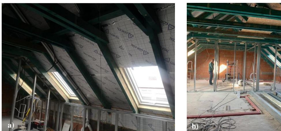
Fig. 3. Pictures from the implementation stage: a) roof insulation, b) general view (Investor's photos, 2020)
