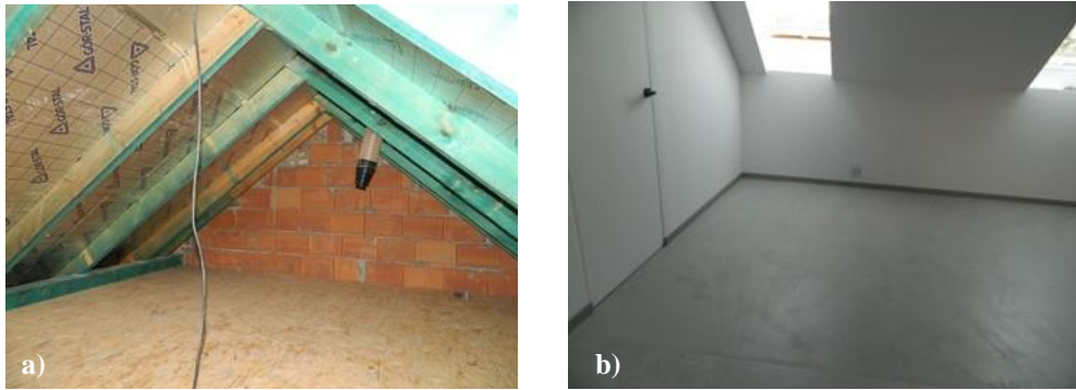
Fig. 4. Pictures after the implementation: a) upper part of the attic, b) lower part of the attic (own photos)
