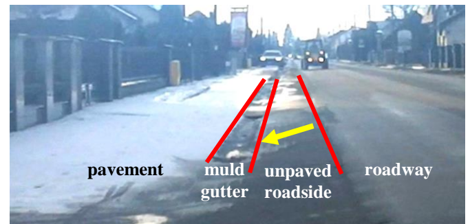
Fig. 7. Incorrect connection of drainage devices
