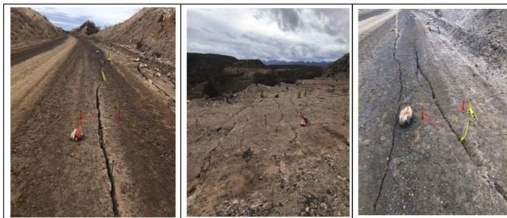
Fig. 5. Observed cracks at M305.
