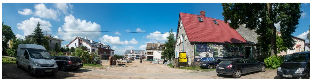
Fig. 9. New housing aggregation under construction with access from Szeroka street. Source: photo by Waldemar Marzęcki
