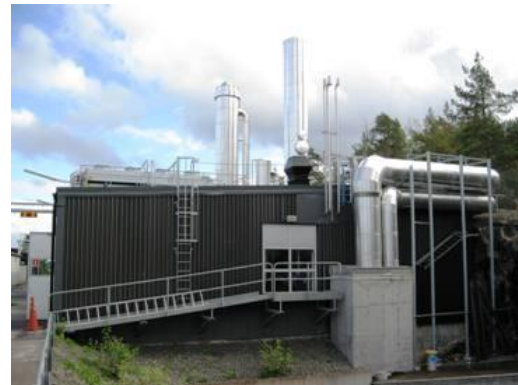
Photo 3. Waste water treatment plant in Stockholm, Sweden (Source: SL, Sweden)
