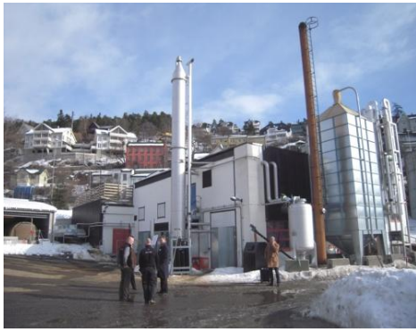
Fot. 4. Biogas upgrading installation in Oslo, Norway
