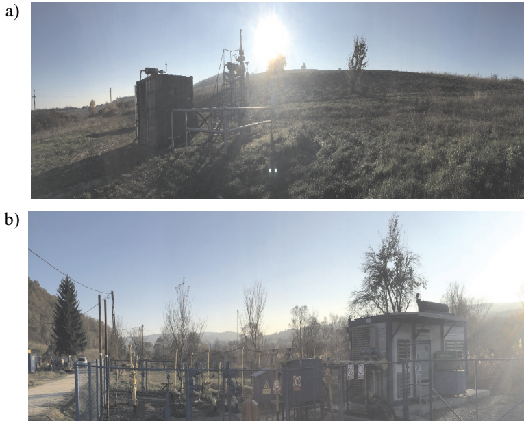
Fig. 5. Wellhead compressor (a) and group compressor (b) in Laslau Mare field
