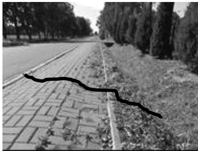
Fig. 7 Deformation of sidewalk due to collapse of ditch wall
