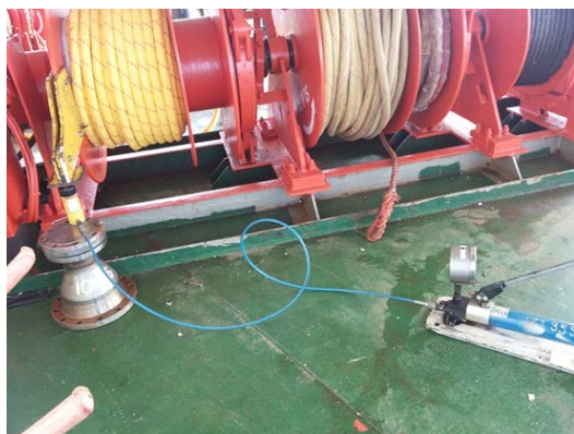
Figure 5. Winch brake test and calibration performed on chemical tanker.
