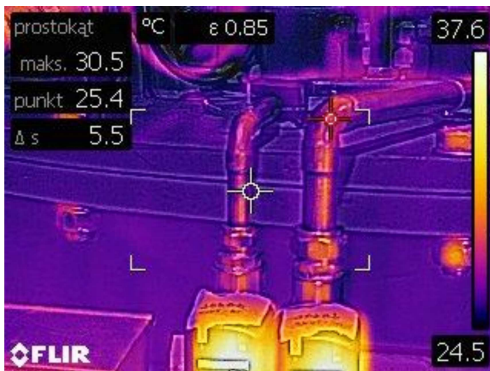
Fig. 4. Thermographic investigation of the cooling sub-system.
