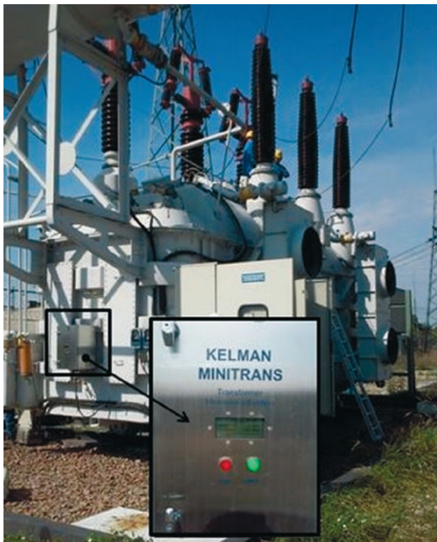
Fig. 2. Monitoring system of water and gas content in oil in 160 MVA autotransformer
