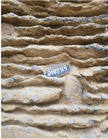
Photo 7. Inlaid works in rubble concrete - street name plaque found in excavation; source: the author
