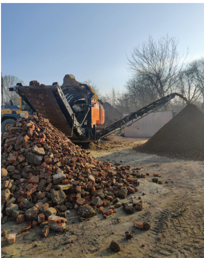
Photo 5. Separation of rubble from loose fractions of excavated material on site using a drum sorter, March 2022; source: Marcin Maraszek
