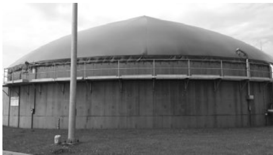
Figure 1. Large-scale semi-buried digester located in north-eastern Poland
