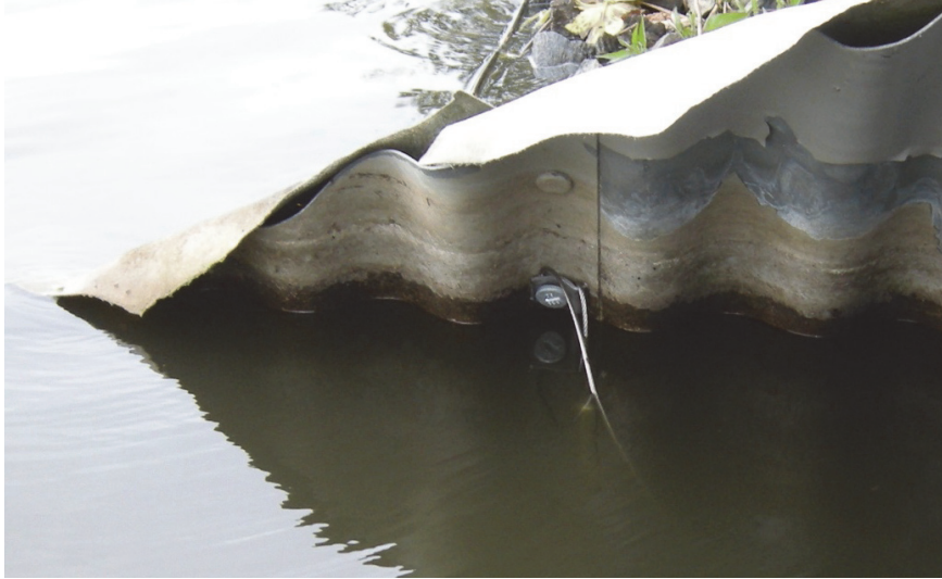
Figure 5. Cathodic protection anodes attached to a culvert
