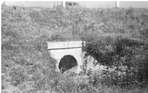
Fig. 1. Road-bed and pipe culvert at km 122+629 of Moscow-Voronezh motorway. Pipe diameter 0.75 m
