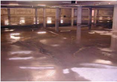
Fig. 1. Leaking floor in an underground parking house due to ignoring the effect of imposed deformation
