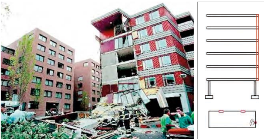
Fig. 4. Progressive collapse of a series of balconies in a high rise building, Maastricht 2003
