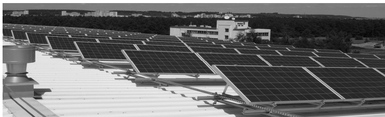
Fig. 1. PV installation on Frosta roof in Bydgoszcz [foto of Authors]
