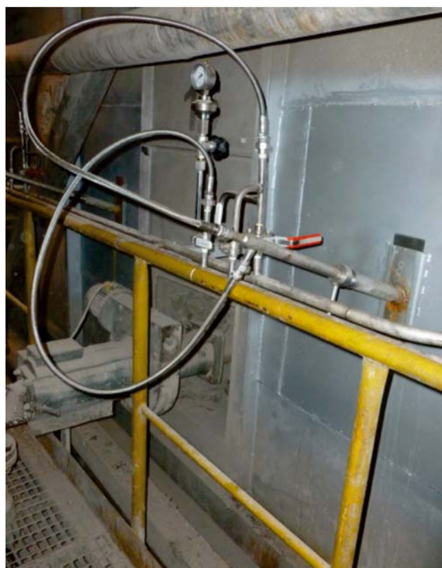
Figure 2. Photo of an injection lance installed in the boiler wall
