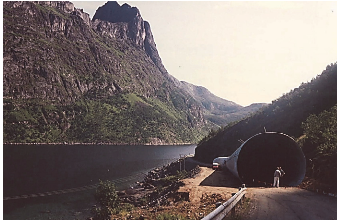
Figure 1. A 6.47 m span flexible avalanche protection culvert built in 1988 in Troms, Norway [1]
