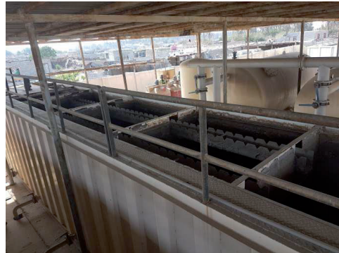
FIGURE 1. Al-Eskan package water treatment plants
