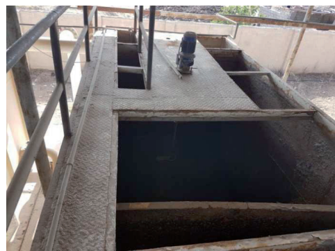
FIGURE 2. Mechanical flocculator in EPWTP
