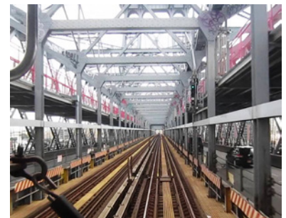
Kratownica i torowisko mostu Williamsburg, fot. YouTube: Riding a J NYC Subway Train across the Williamsburg Bridge to Brooklyn
