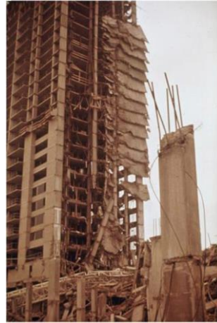
Fig. 4. The view of the Skyline Plaza building in Virginia after the progressive partial collapse of its central part as a result of punching in support zones of flat ceiling slabs
