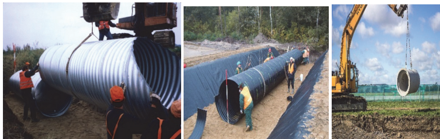
Fig. 6. Three pipes used to build a culvert– a) CSP galvanized b/ CSP in TC c) RCP (reinforced concrete pipes)
