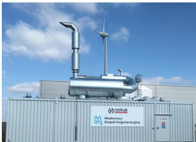
Fig. 4. The cogeneration unit with Perkins 4016-61TRS2 industrial gas engine equipped with the WUZG system at customer site in Gaj Oławski
