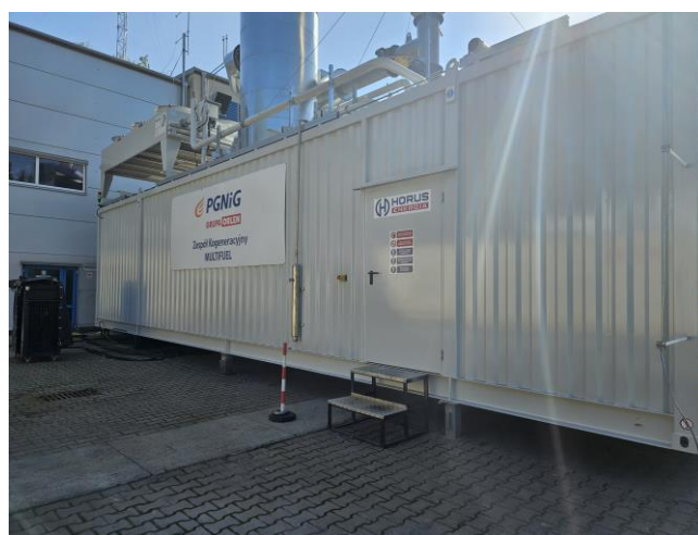
Fig. 6. The containerised cogeneration unit with the Perkins 4016-61TRS2 industrial gas engine at Horus-Energia industrial engines test facility
