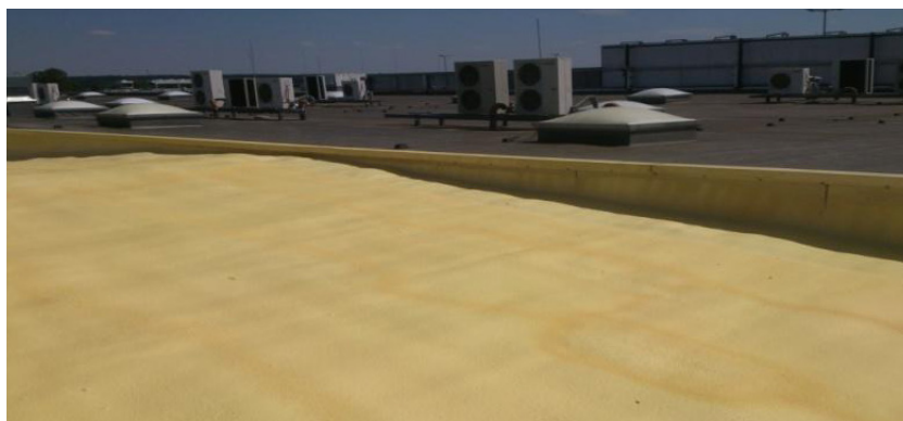
Fig. 2. The roof after the restoration with the use of the plastic foil. Higher level of aesthetics. Source: R. Pilch
