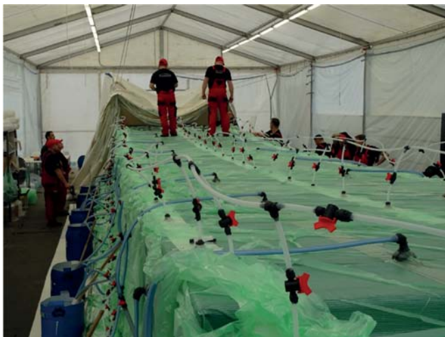
Fig. 2. Preparation to infusion of a large-size object - footbridge span of Fobridge grant
