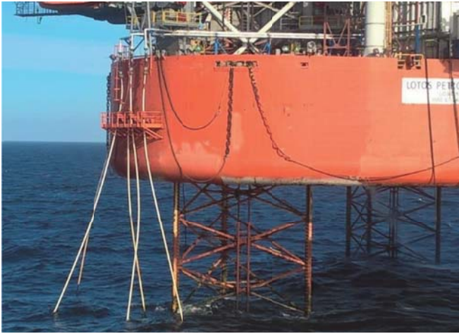
Fig. 14. CT 4" pipes operating in the water injection system on the LOTOS Petrobaltic platform
