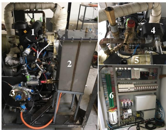
1 – SI engine, 2 – Lubricating oil tank, 3 – Pressure reducer, 4 – Low temperature heat exchanger, 5 – High temperature heat exchanger, 6 – Control cabinet.
