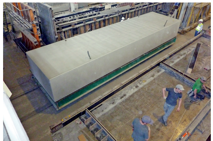
Fig. 11. Placing the pontoon on the adjacent working platform following removal of formwork
