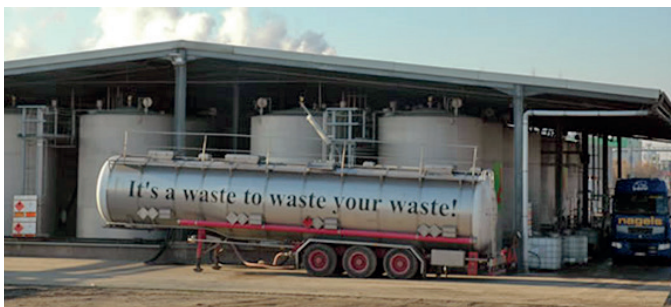
Fig. 3. Courtesy of De Neef Chemical Processing, Belgium
